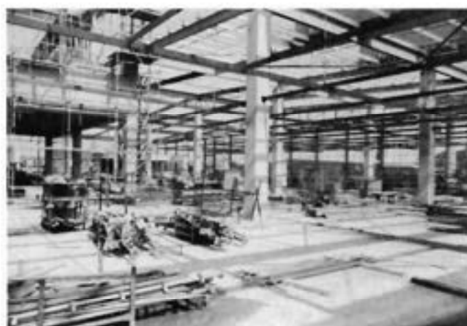
Fig 12. Services subframe in the sorting office
