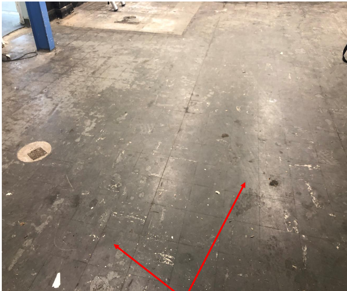
Asbestos Thermoplastic Floor Tiles with Asbestos Adhesive Backing(s) – See Recommendations
