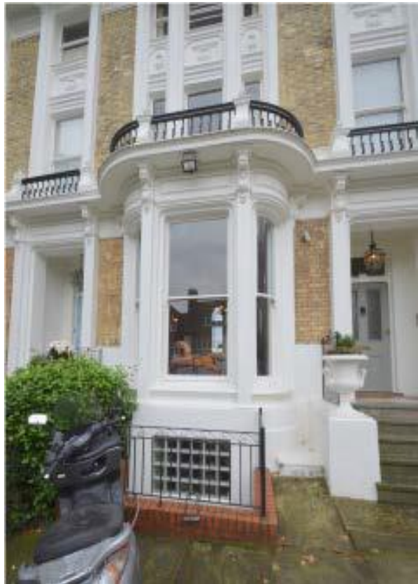
Image 5: Existing railings around the central lightwell to be replaced with railings to match the existing railings either side of the front door steps (see image 6) in finish, style, material and colour.
