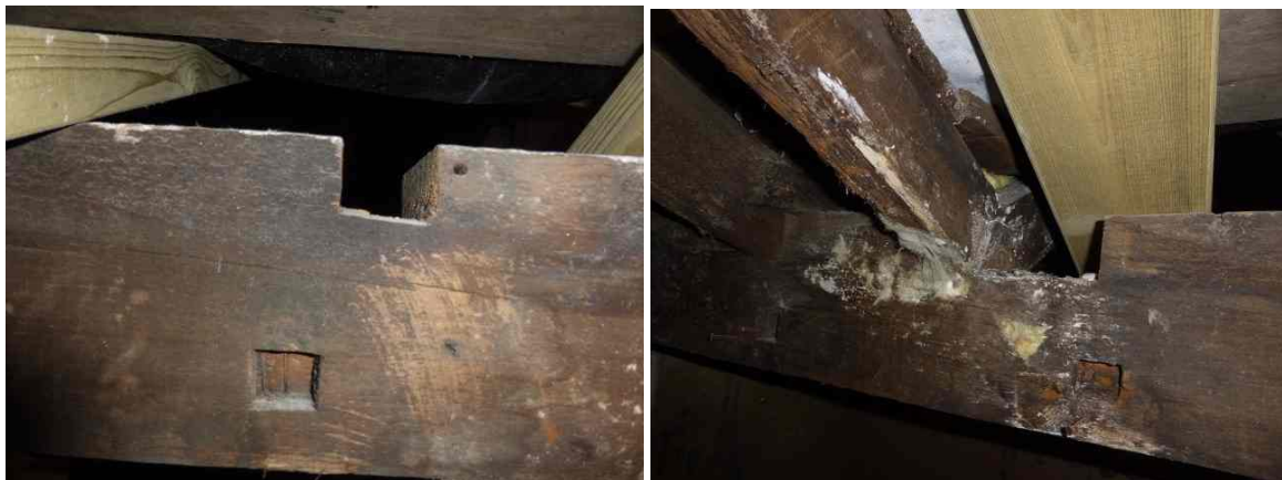
Figs. 11 - 12 Notching revealed in opening up compromising integrity of the valley beam
