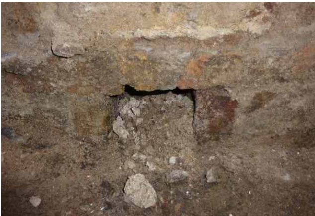
Fig. 5 Below slab vent to external cavity still semi-blocked with concrete
