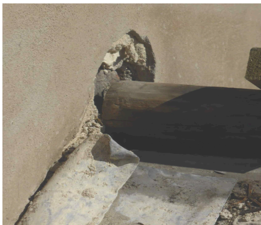
Fig. 16 Original timber lead roll adjacent to party wall uncovered following removal of the terrace
