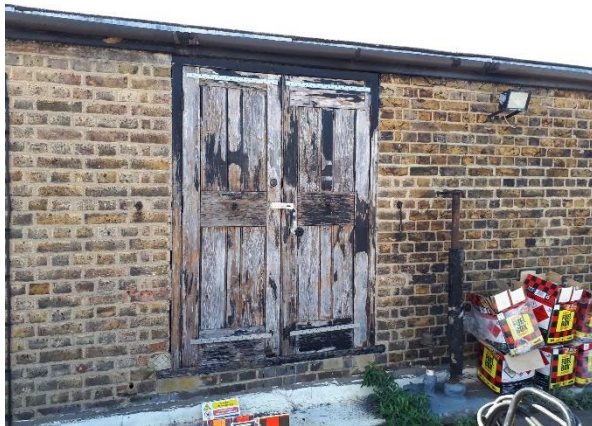
Existing rotten timber double door set to plant room at roof level. Propose to replace with new fire rated steel powder coated double door set.
