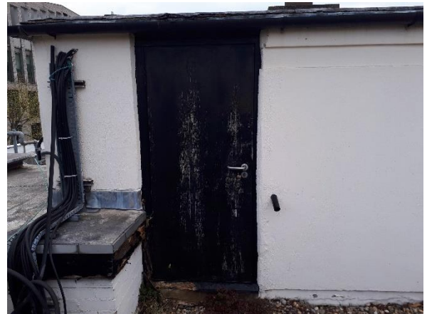
Existing rotten timber door set to plant room at roof level. Propose to replace with new fire rated steel powder coated single door set.
