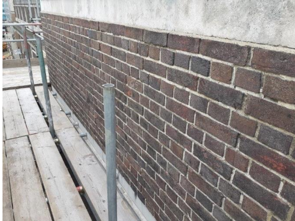
Existing defective pointing to external elevation.
