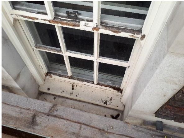
Example of extent of timer decay to sash windows at third floor level.
