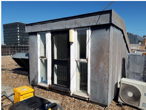
Existing rotten timber door set and single glazed side panels. Propose to replace with new double-glazed powder coated aluminium type double door set.
