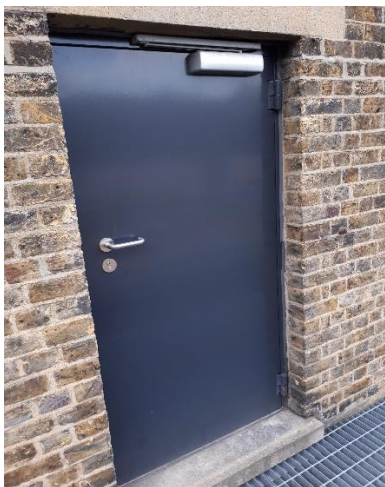
Existing fire rated steel door set installed at roof level. We propose to replace the timber doors to the plant rooms to match this.
