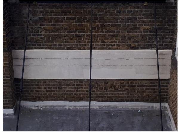
Close up showing cracked and defective render to the panels within Roof 1.
