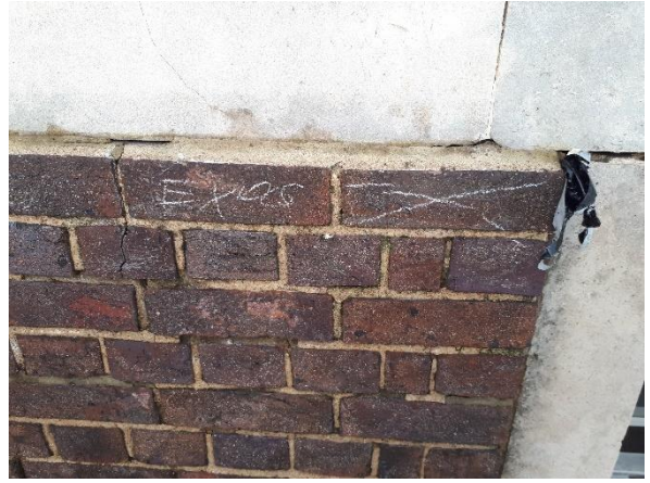
Evidence of cracked brickwork and movement due to the corroded steel frame behind.
