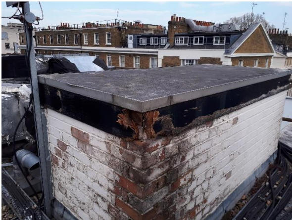
Paint finish to roof 13 deteriorating. We propose to prepare and redecorate.
