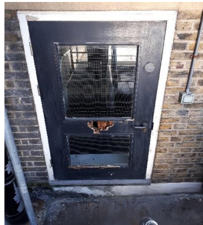
Existing rotten timber door set to roof top plant area. Propose to replace door set with new hardwood fire door. Configuration of glazing to match existing.
