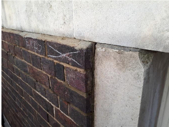
Evidence of brickwork being pushed out due to the corroded steel frame behind.
