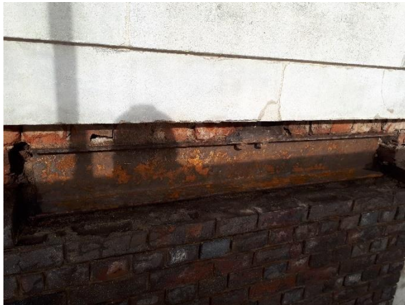
Corroded steel frame behind brick panel.
