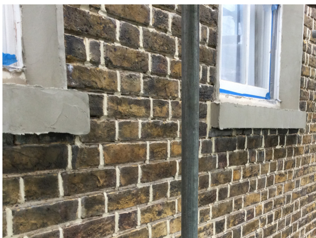
Figure 5: Cementitious coating of cills/reveals at 2nd floor; Brick pointing has not proceeded to lower floors.
