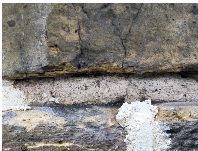
Figure 6: Preceding lime mortar sample visible
