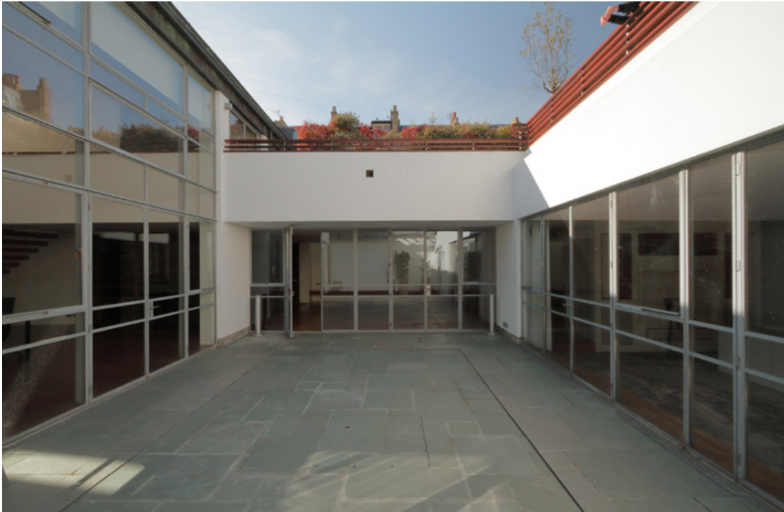
[C] View of existing pool courtyard and ancillary wing structure, due north-west [image source: Author]
