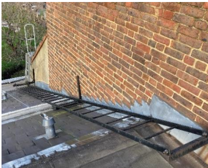
Figure 6: Existing Condemned Roof Ladder 6NS
