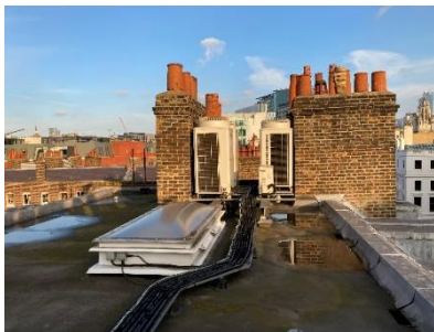
Figure 4: Existing Felt Roof – 5 New Square E
