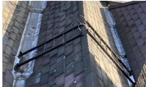
Figure 7: Existing Condemned Roof Ladder 5NS
