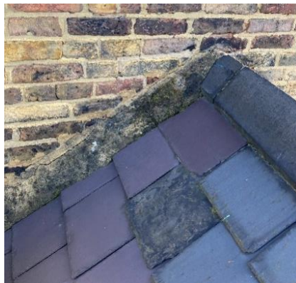
Image 9: Failed rendered plinth detail
