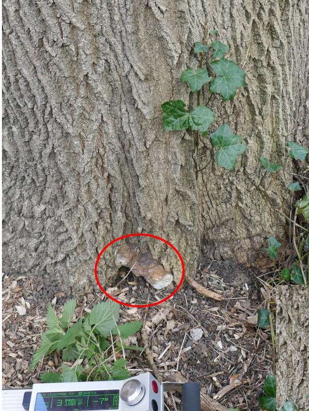
1) Cavity opening at the base of the larger S trunk with Ganoderma bracket by the opening
