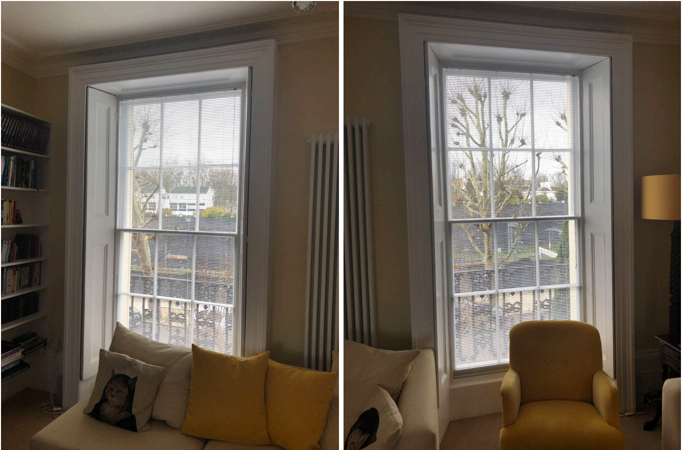
Figure 6: Internal view of 2no. windows in the living room at first floor
