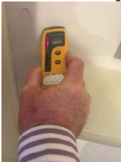
Moisture meter readings suggesting rising dampness
