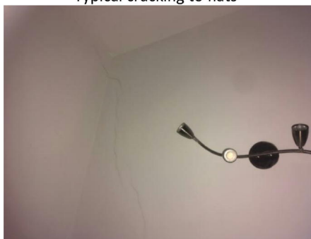
Typical cracking to flats
