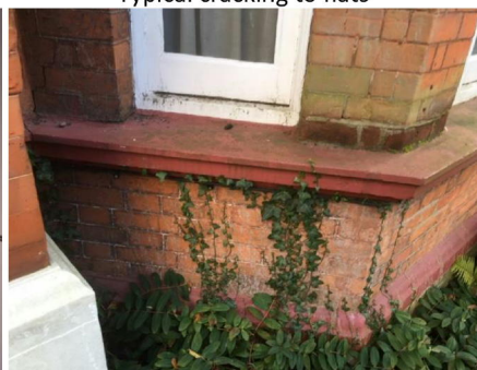
External cracking to bay
