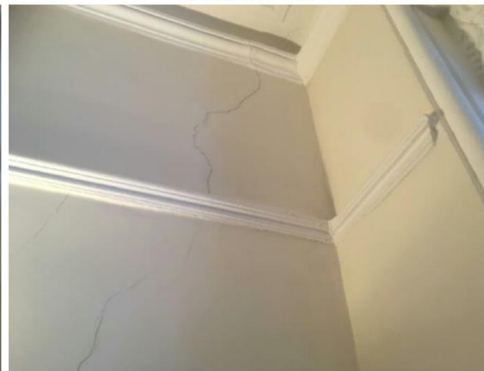
Typical cracking to flats
