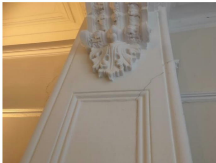
Typical cracking to flats
