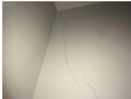
Typical cracking to flats
