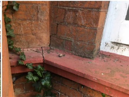
External cracking to bay
