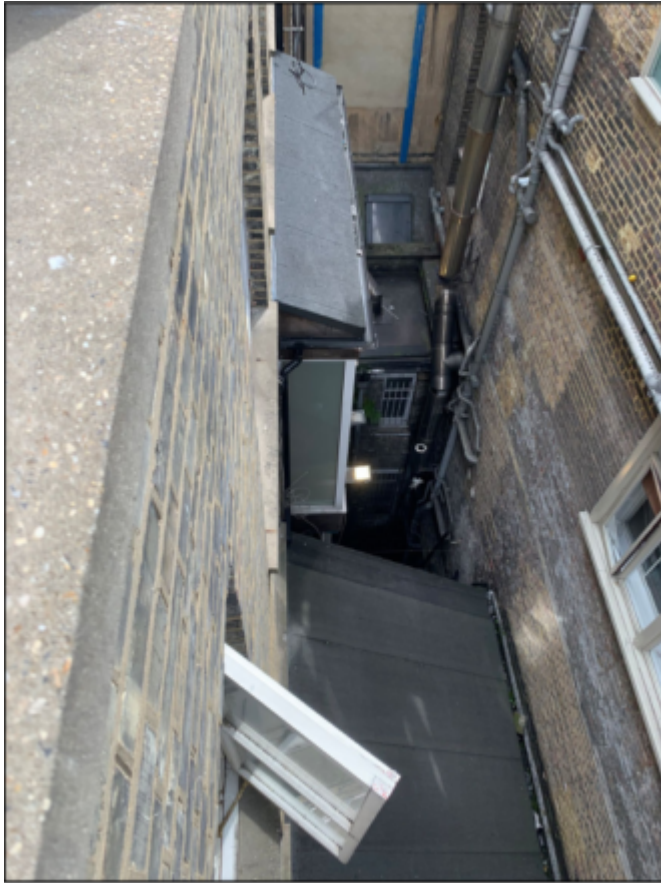
Photo 4 (above): Close-up view of existing first floor rear bay window extension to be demolished
