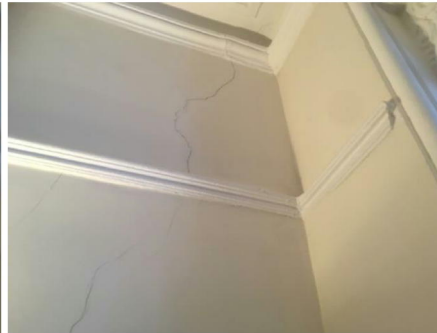
Typical cracking to flats
