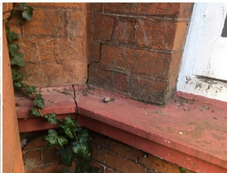
External cracking to bay
