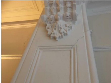
Typical cracking to flats
