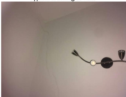
Typical cracking to flats
