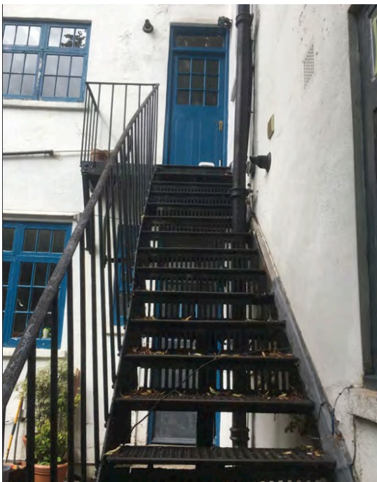
poor integration of stairs has a rainwater pipe running through it.
