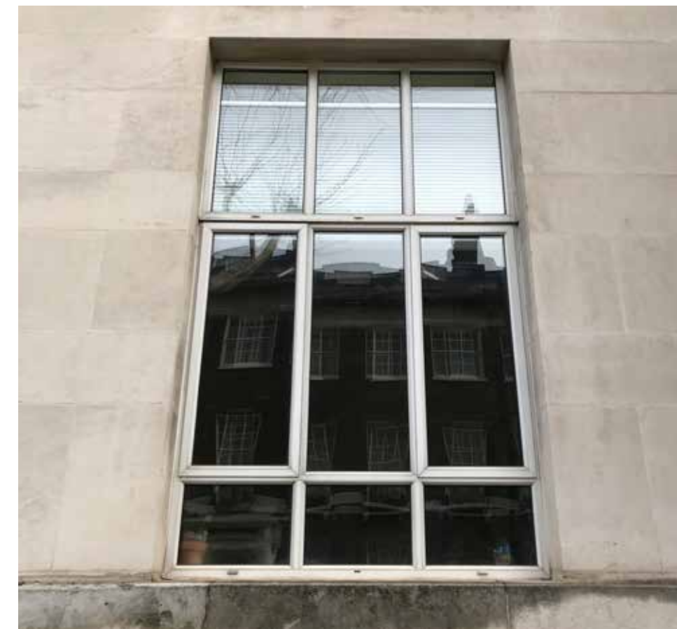
03. Typical double-glazed non-thermally broken aluminium windows with slim glazing bars located within glass units.
