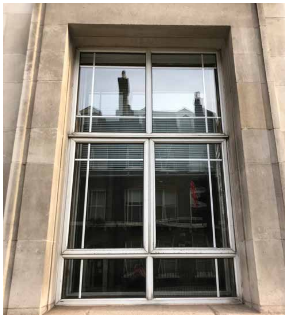
02. Typical double-glazed non-thermally broken aluminium windows with slim glazing bars located within glass units.
