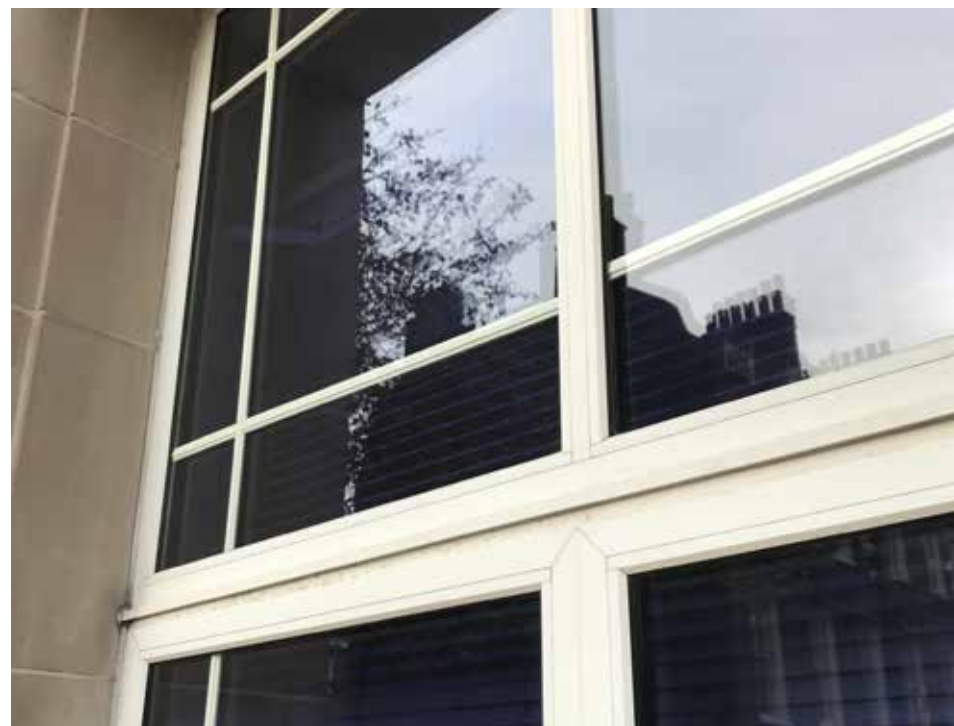
01. Close up of slim glazing bars located within double-glazed non-thermally broken aluminium framed windows.
