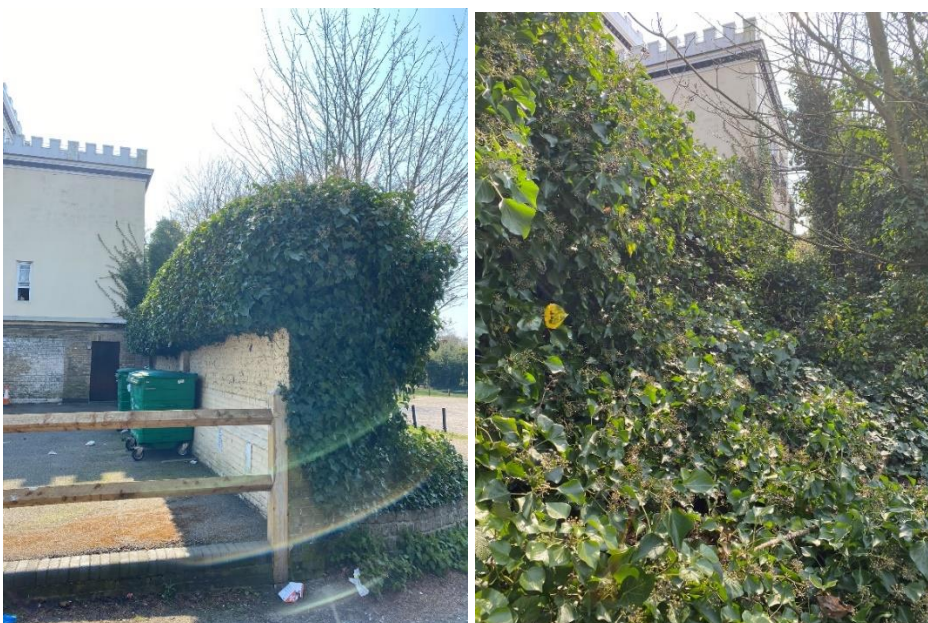
Figure 4.3 The ivy clad wall (left) and tree/scrub line of the next door car park (right)
