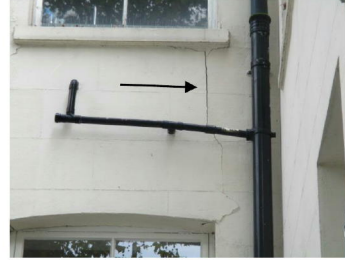
Cracking to rear elevation
