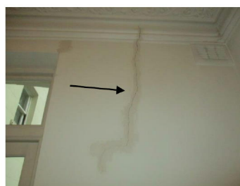
Cracking in ground floor dining room
