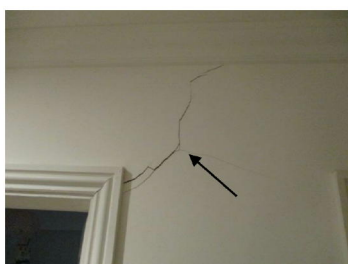
Cracking in basement hallway
