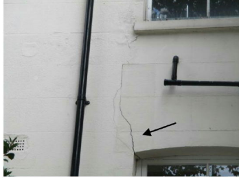
Cracking to rear elevation
