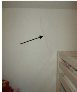
Cracking in basement bedroom
