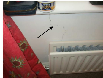
Cracking in upper flat rear study
