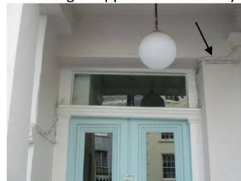
View of historic distortion and recent cracking above front door
