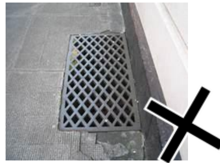
Grille – not acceptable
