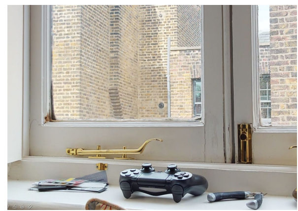
EXISTING NON-ORIGINAL CASEMENT WINDOWS IN VERY POOR CONDITION.
