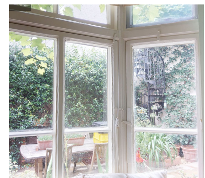
EXISTING NON-ORIGINAL CASEMENT WINDOWS IN POOR CONDITION.
