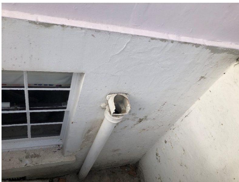
Figure 4: Broken Ventilation Pipe
