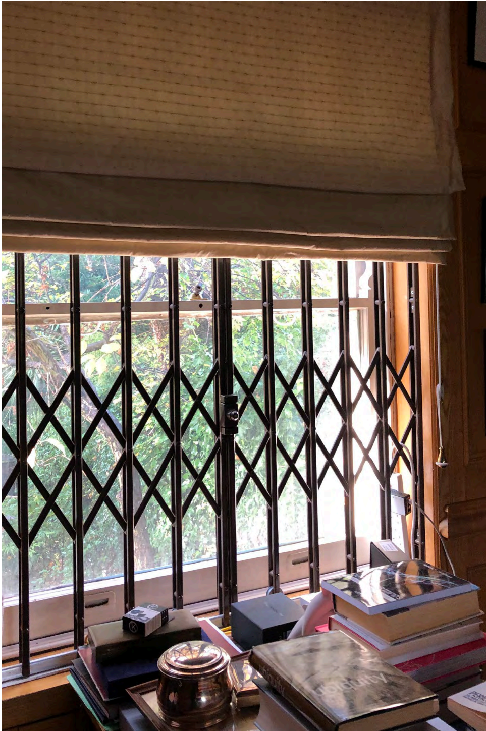
Figure 16: Internal view of the left-hand side window in the office at ground floor level
