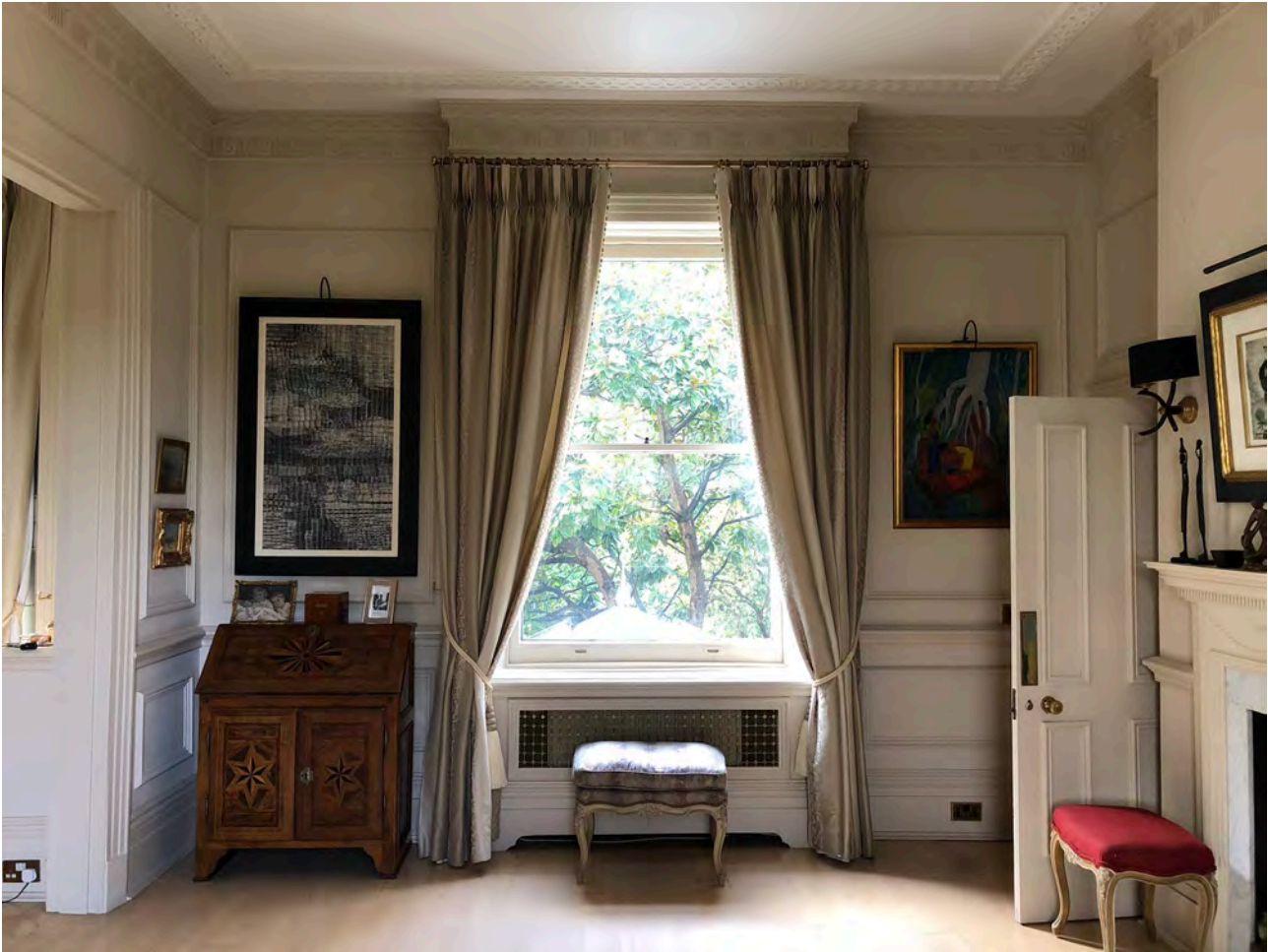
Figure 13: Internal view of the left-hand side window in the lounge at ground floor level
