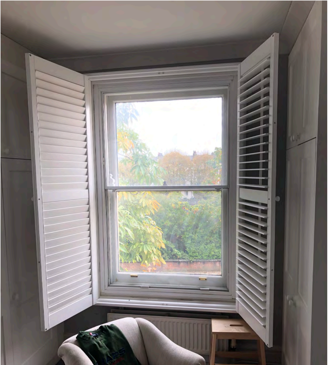
Figure 18: Internal view of the right-hand side window in the first floor bedroom
