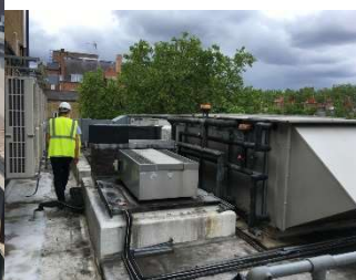
Figure 3, Western View within plant compound
