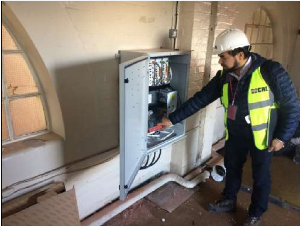
Photograph 5 – An example of a CP control cabinet [TR]
