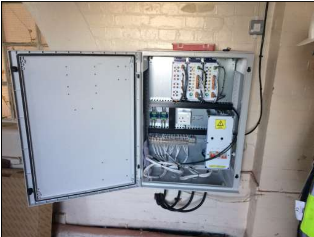
Photograph 6 – Inside of a CP control cabinet [TR]
