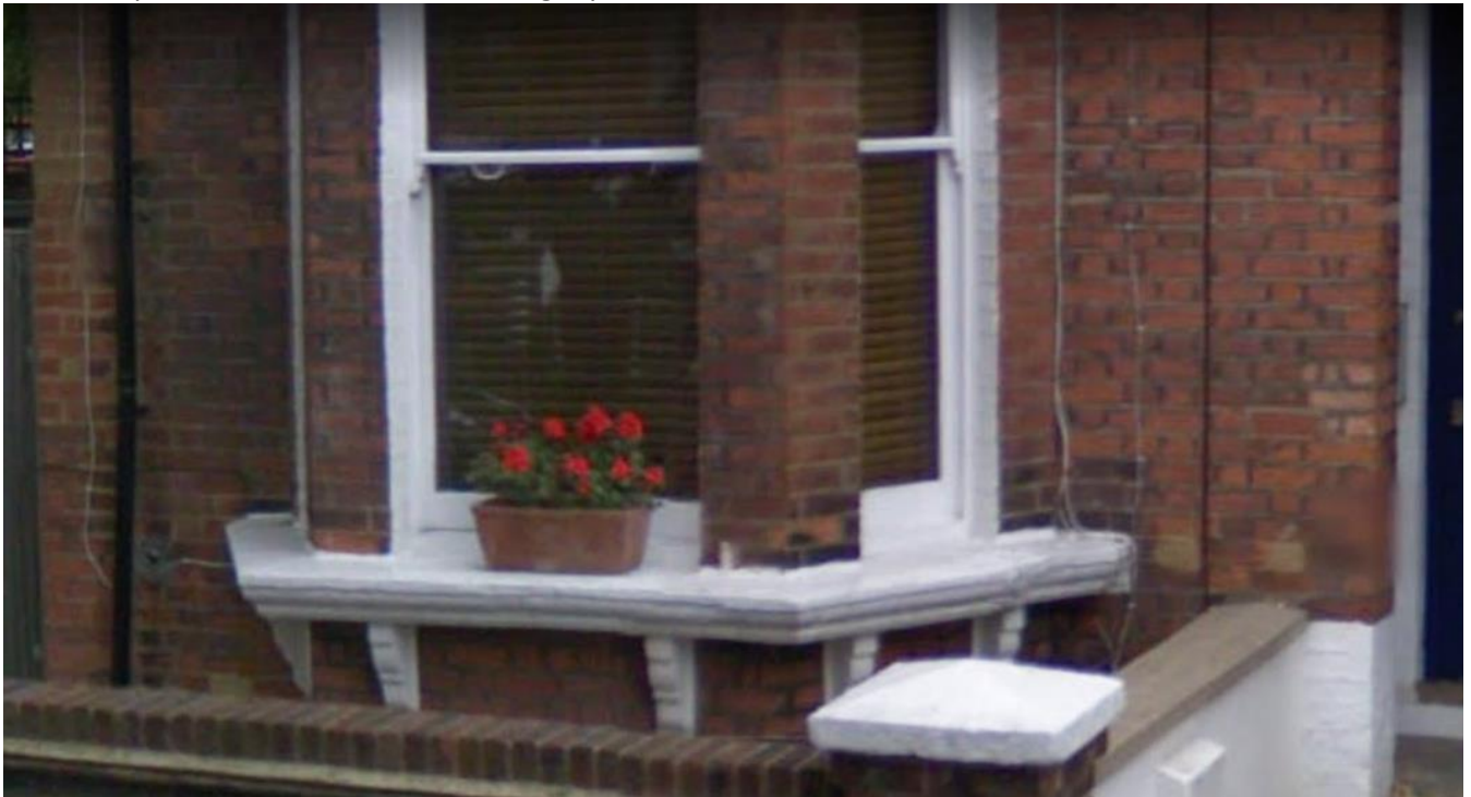
- tell-tale gap under the left side of the sash window when fully closed
