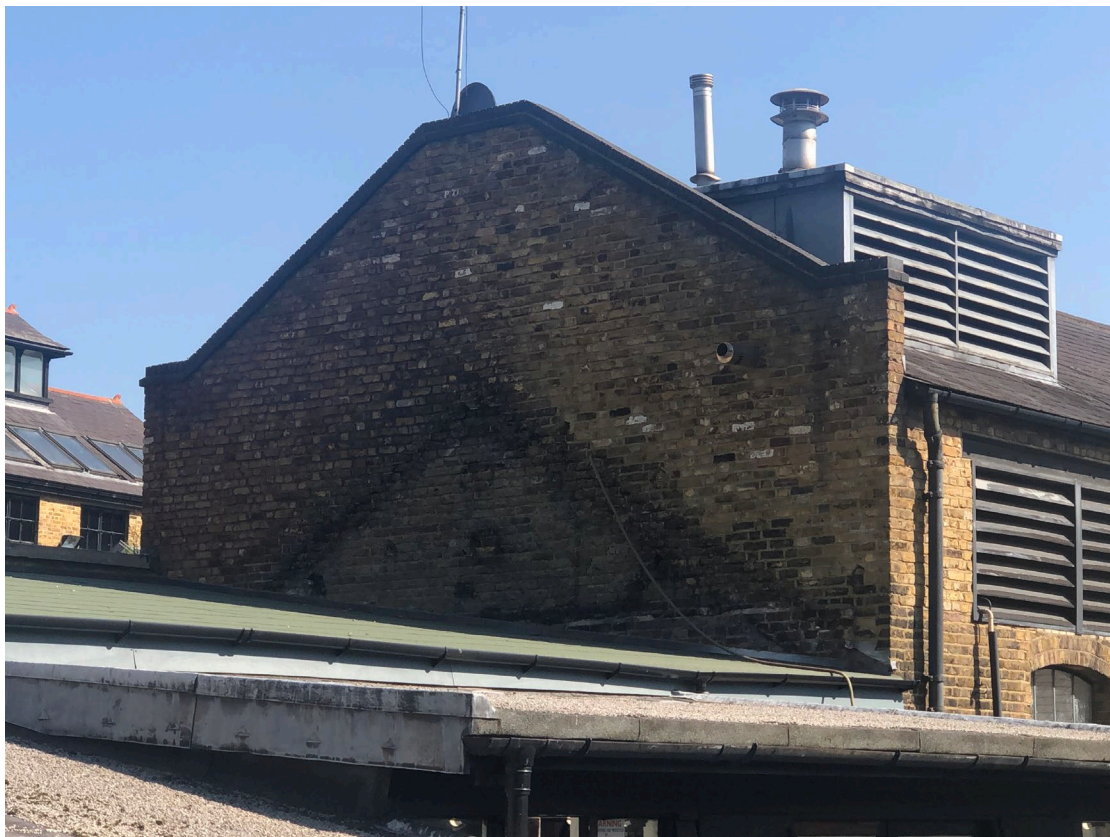
Profile of burnt roof over temporary construction
