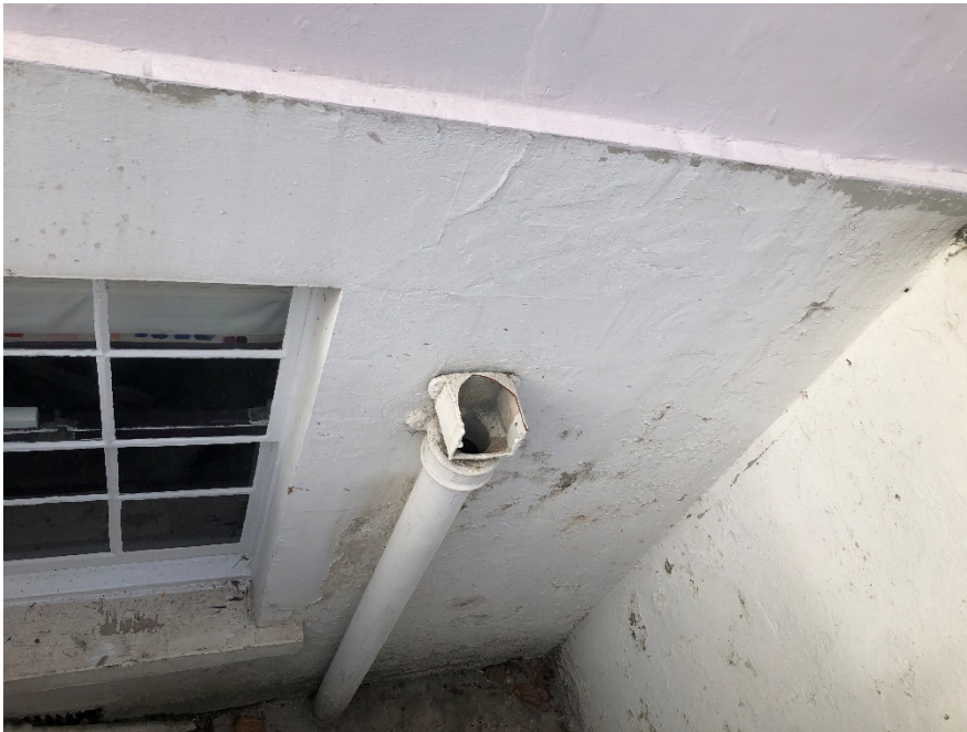
Figure 5: Broken Ventilation Pipe
