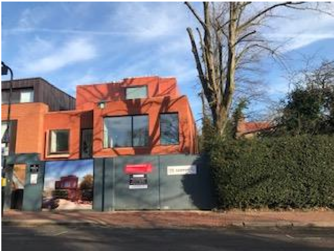
2. (above): View towards front elevation of 36 Redginton Road which is under construction (38 Redginton Road is on left)
