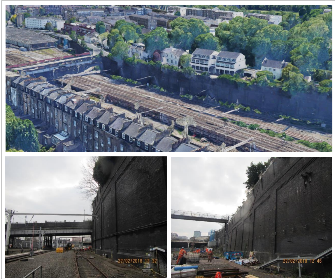
Figure 9 Top: Aerial view showing the existing western PVE wall (Google Maps). Bottom: Southward view of the existing retaining wall toward Mornington Street Bridge (left) and view south of Mornington Street Bridge (right).
