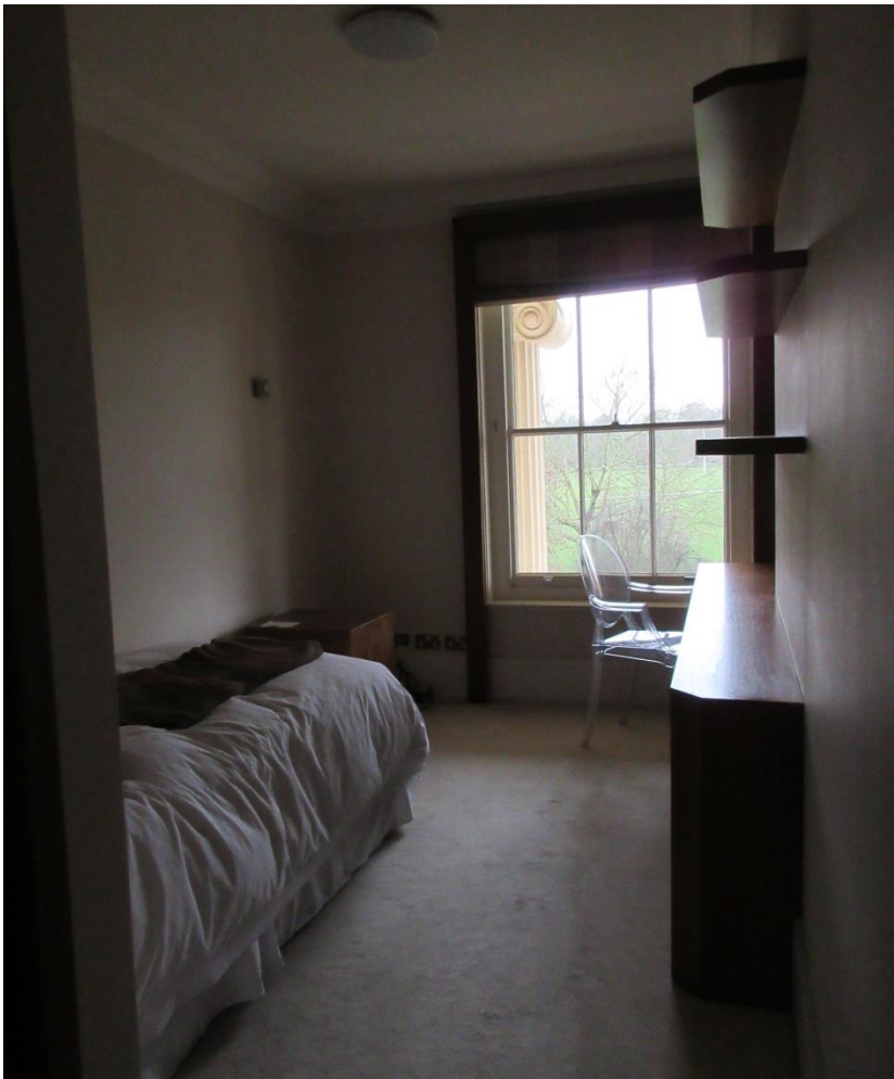
Figure 17: The existing study was created during the 1960s subdivision of the original No. 15; there is no visible evidence for the chimneybreast which would have been located within the party wall (right).
