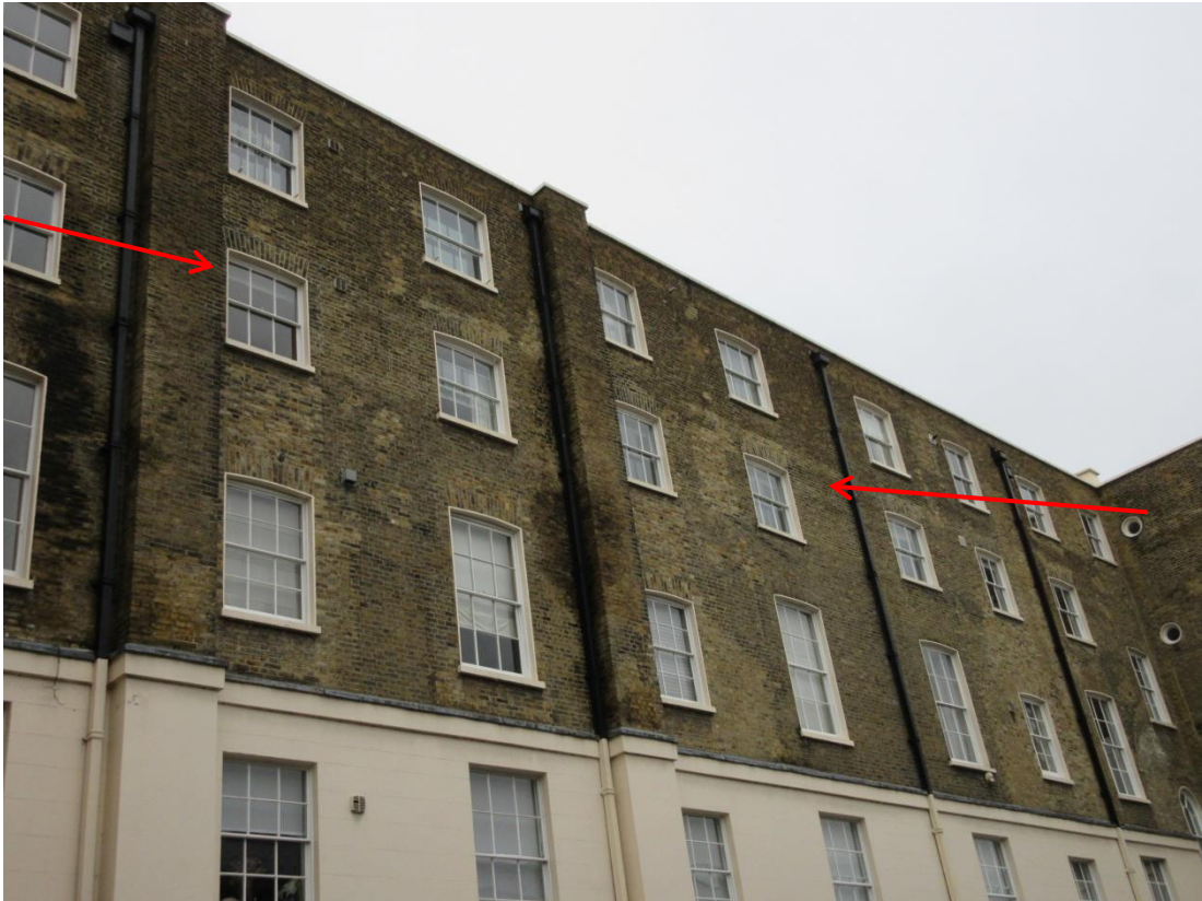
Figure 14: The rear elevation of the subject site at second-floor level; the scarring of substantial previous alterations is evident across the elevation.
