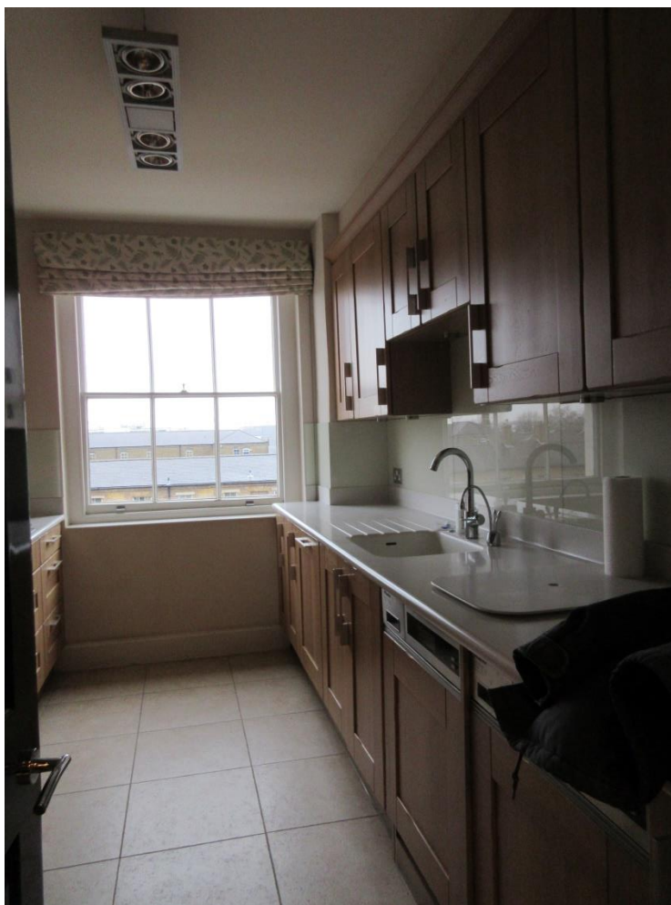
Figure 19: The existing early 1960s galley kitchen within the infilled stairwell area at the rear of No. 15.
