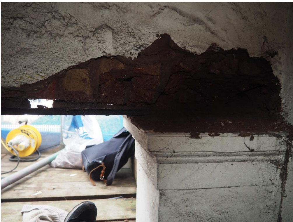
Plate 4a&b: Exposed Rusted Plate
