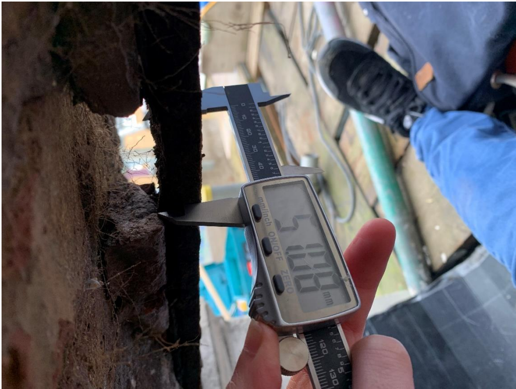
Plate 5a&b: Exposed Rusted Plate
