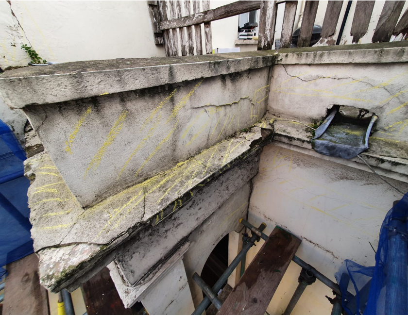
Side view of porch parapet with damaged render
