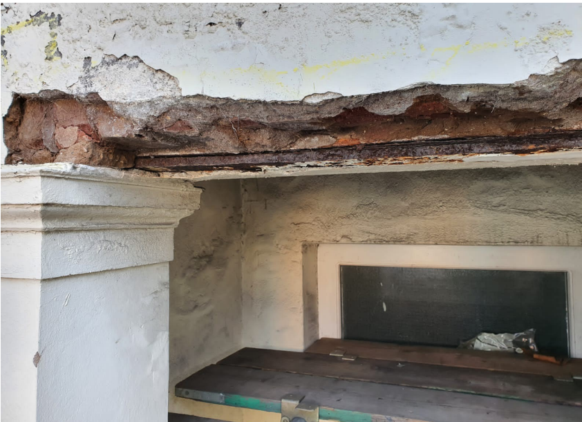
Exposed iron flat showing brickwork above
