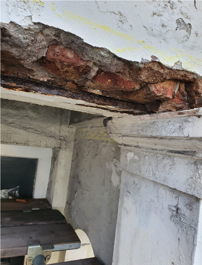
Exposed iron flat showing bearing to column
