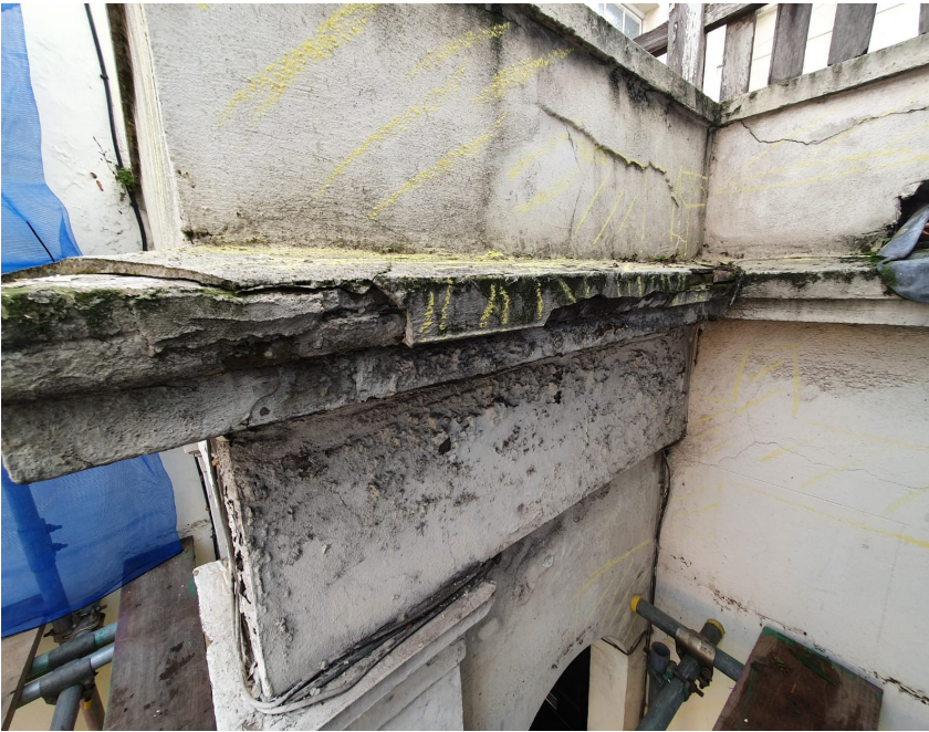
View of porch parapet with damaged render to projecting concrete work
