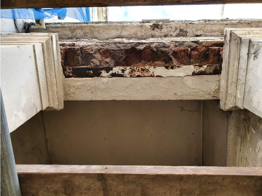
Underside of iron flat following removal of spalled render
