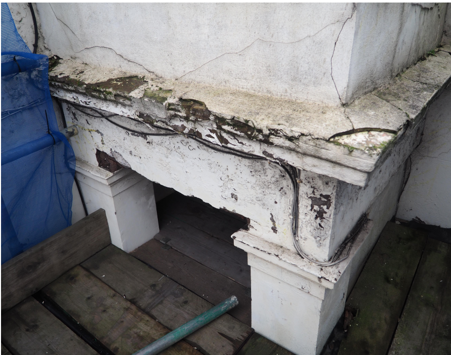
Projecting course showing moulded stonework to left and presumed concrete work to corner section, with spalled and missing render
