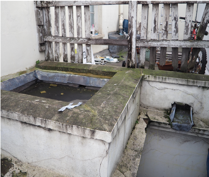
View from above showing asphalt roofing and unclipped flashing
