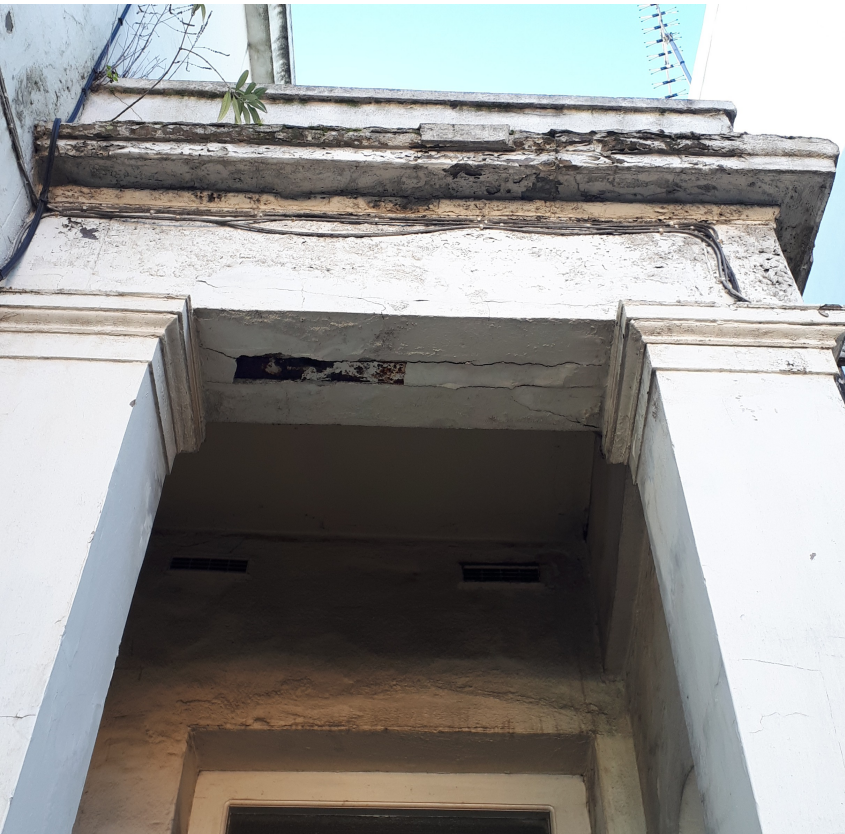
Underside of porch entablature showing spalled render prior to opening up
