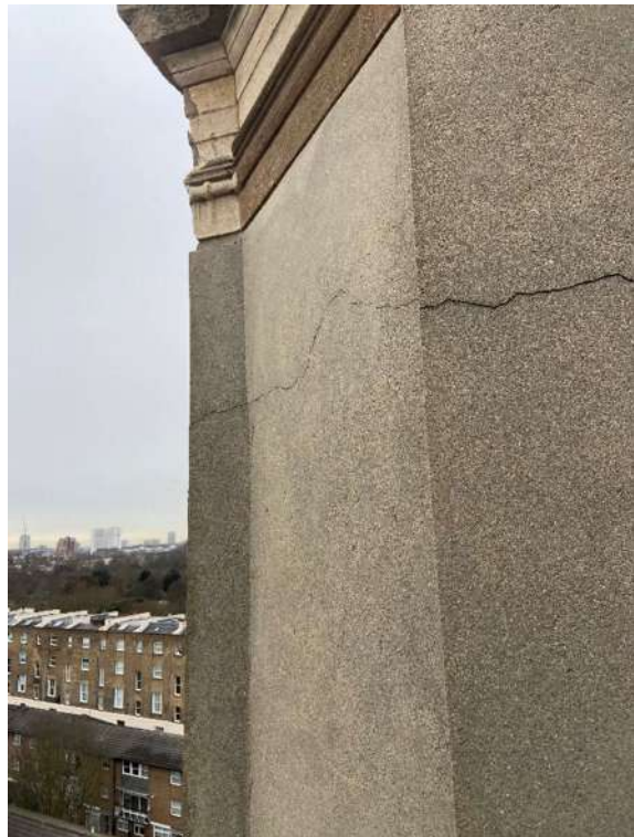
Img 04; horizontal cracking at high level.
