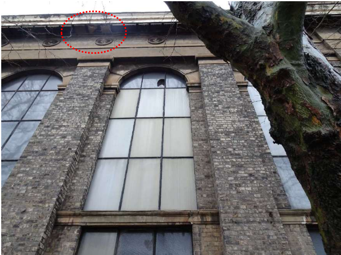
Img 19; rendered cornice on north elevation (liturgical) showing historic failure of rendered 'mutules' (circled)
