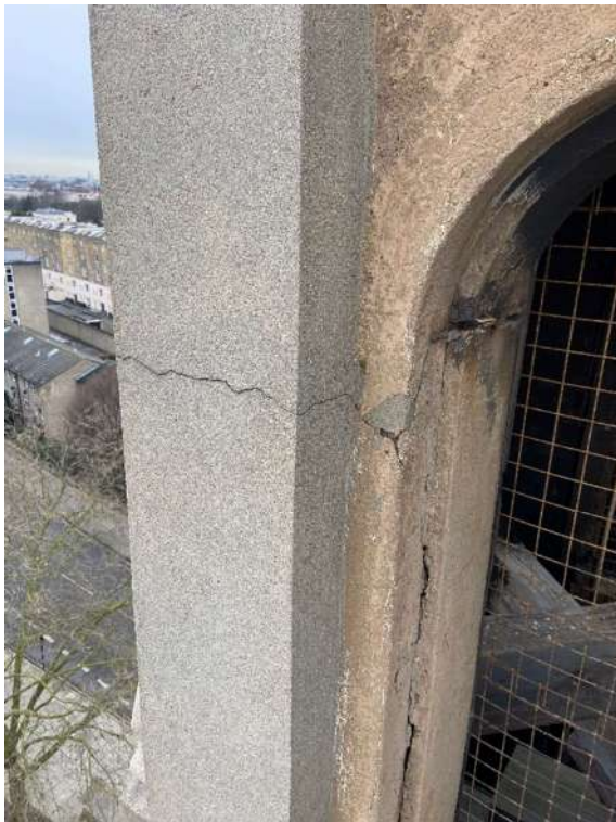
Img 03; cracking through render and repairs
