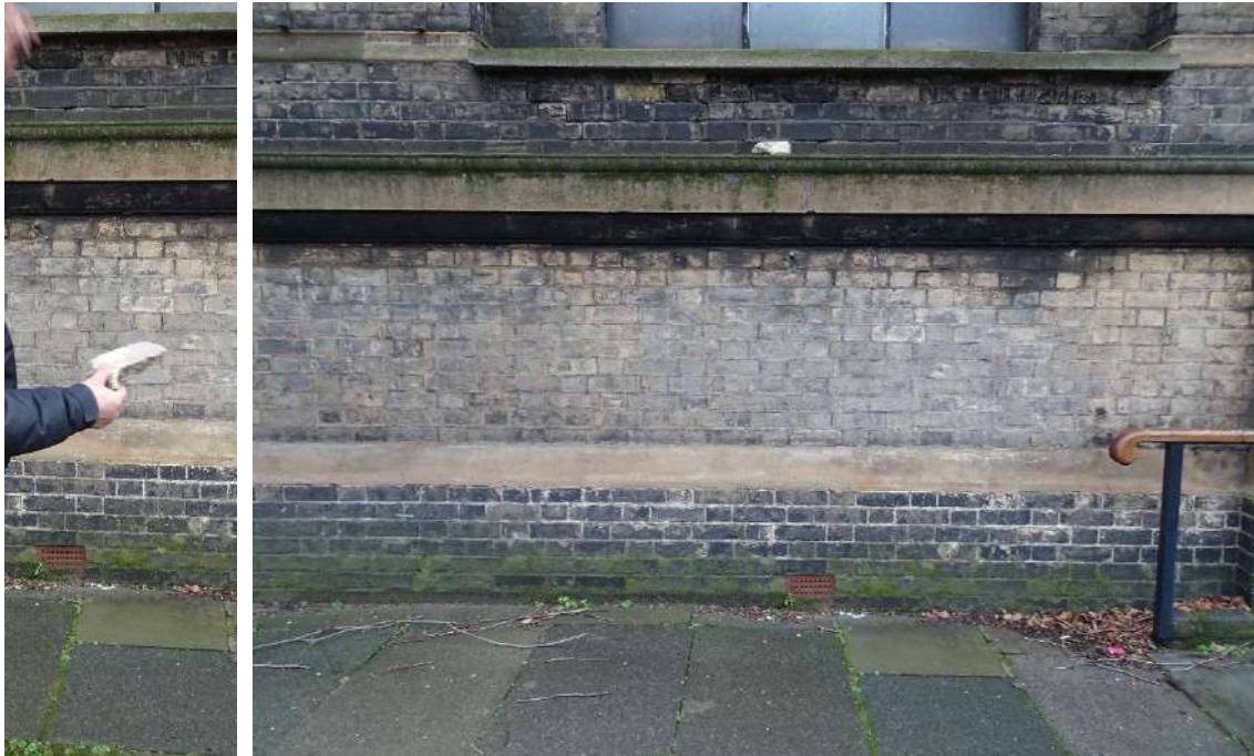
Img 17 and 18; render from debris found on the wall moulding which would have fallen in excess of 10m.
