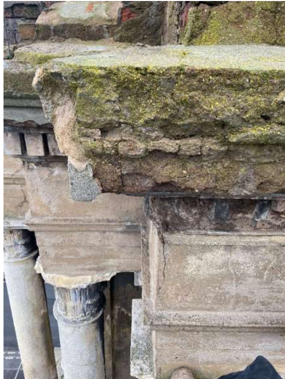
Img 10 and 11; failing render and brick dentils
