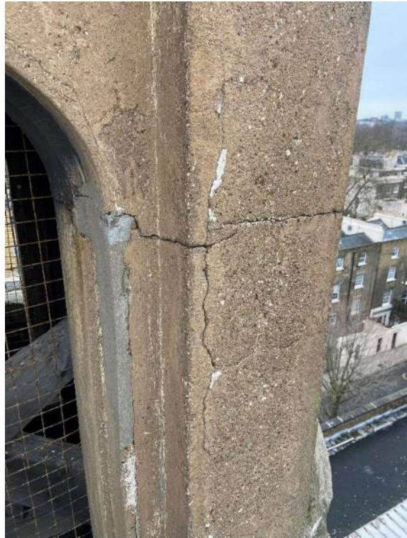
Img 02; cracked render and previous cement repairs
