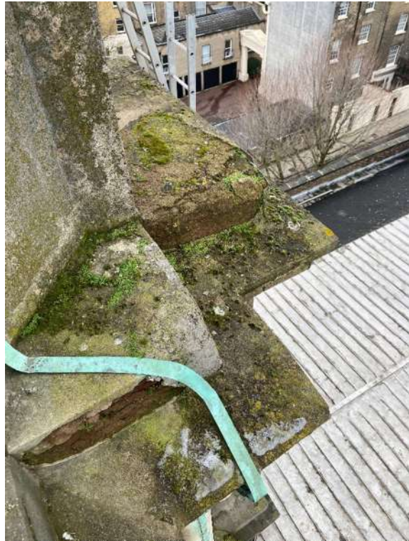
Img 06; general poor condition of render
