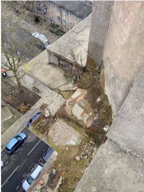
Img 05; failing render on sky-facing elements
