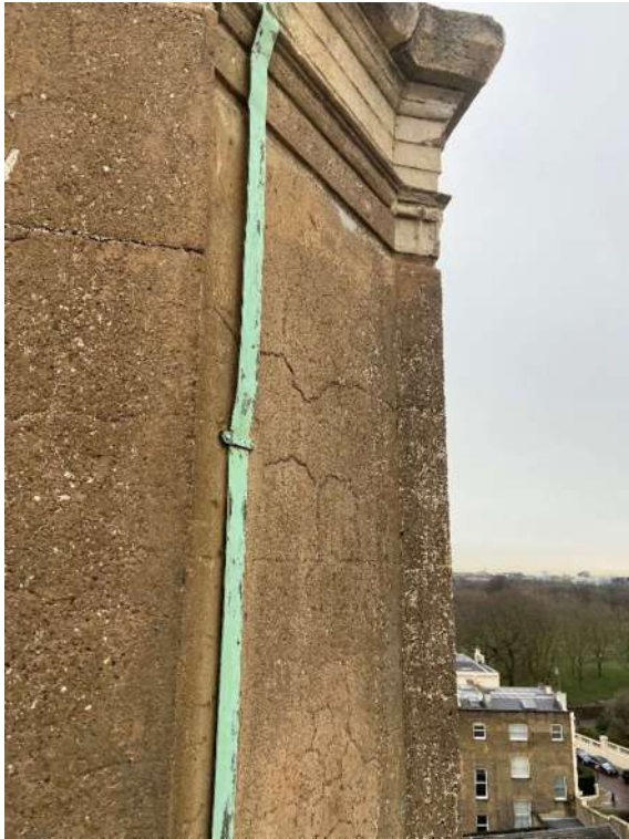
Img 01; cracked render
