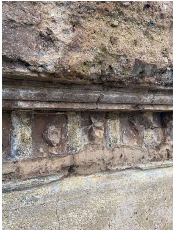
Img 12; close up view of failed brick dentils
