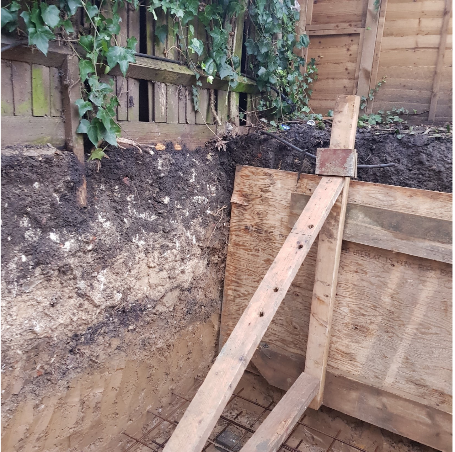
Photograph 01 showing the trench to the rear of the No.25 garden. Note the concrete foundations above the clay and the lack of visible significant roots.
