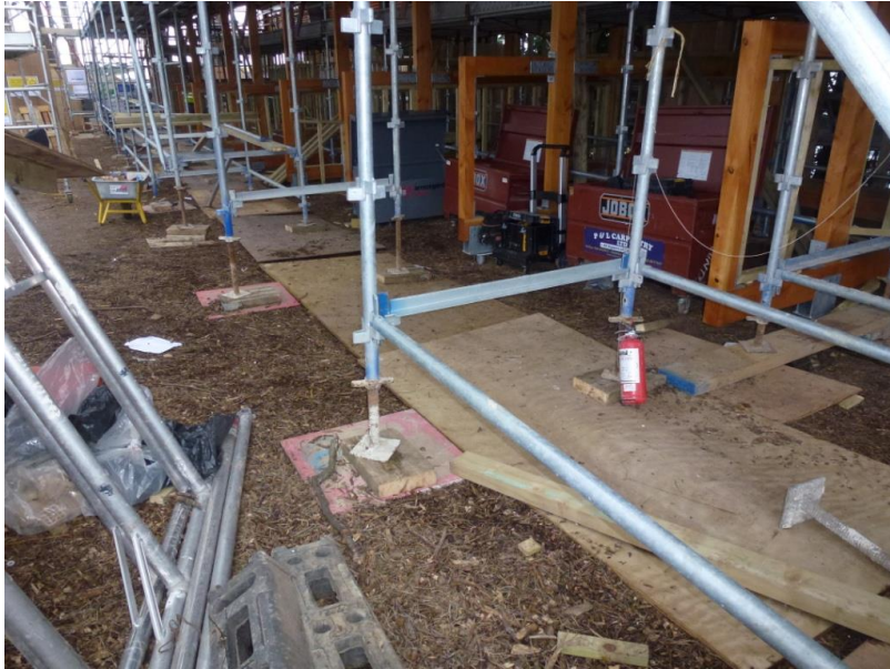
Image 3: Scaffolding within tree protection zones: Scaffolding can be facilitated using blocks placed on ground protection to facilitate erection of the structure and pedestrian walkways without ground compaction.
