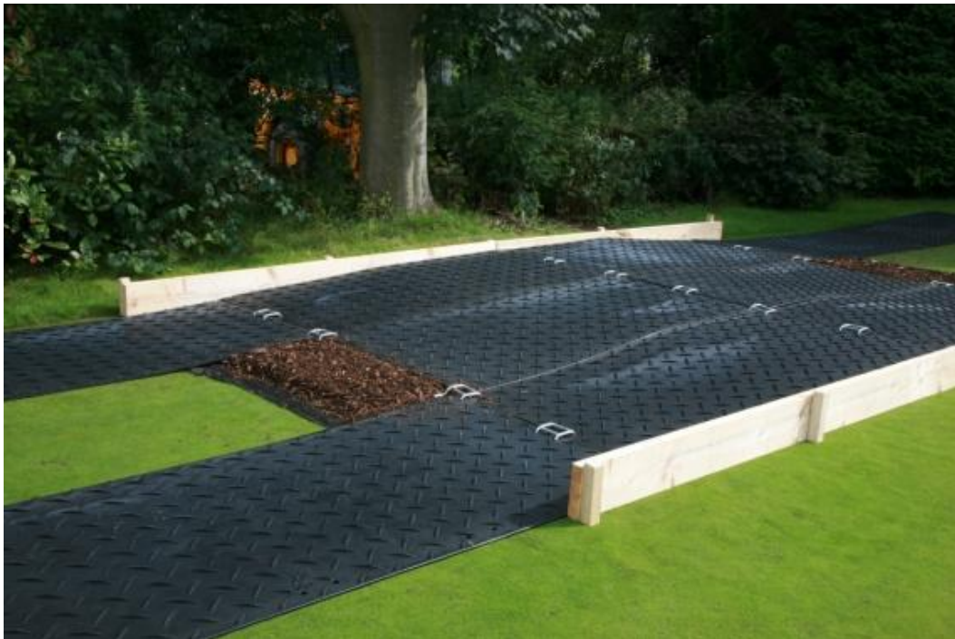
Photo 2: Ground-Guards, installed using a geotextile membrane, ground panels, 150mm deep woodchip and ground panels on top and held in place with edge rails. Please refer to www.ground-guards.co.uk/ for more details.
