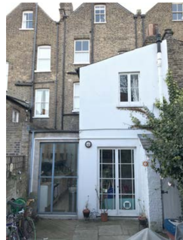
Rear elevation showing non-original openings and side infill extension in poor condition.
