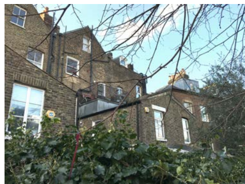
View towards altered rear elevations to the North showing the large water tank.
