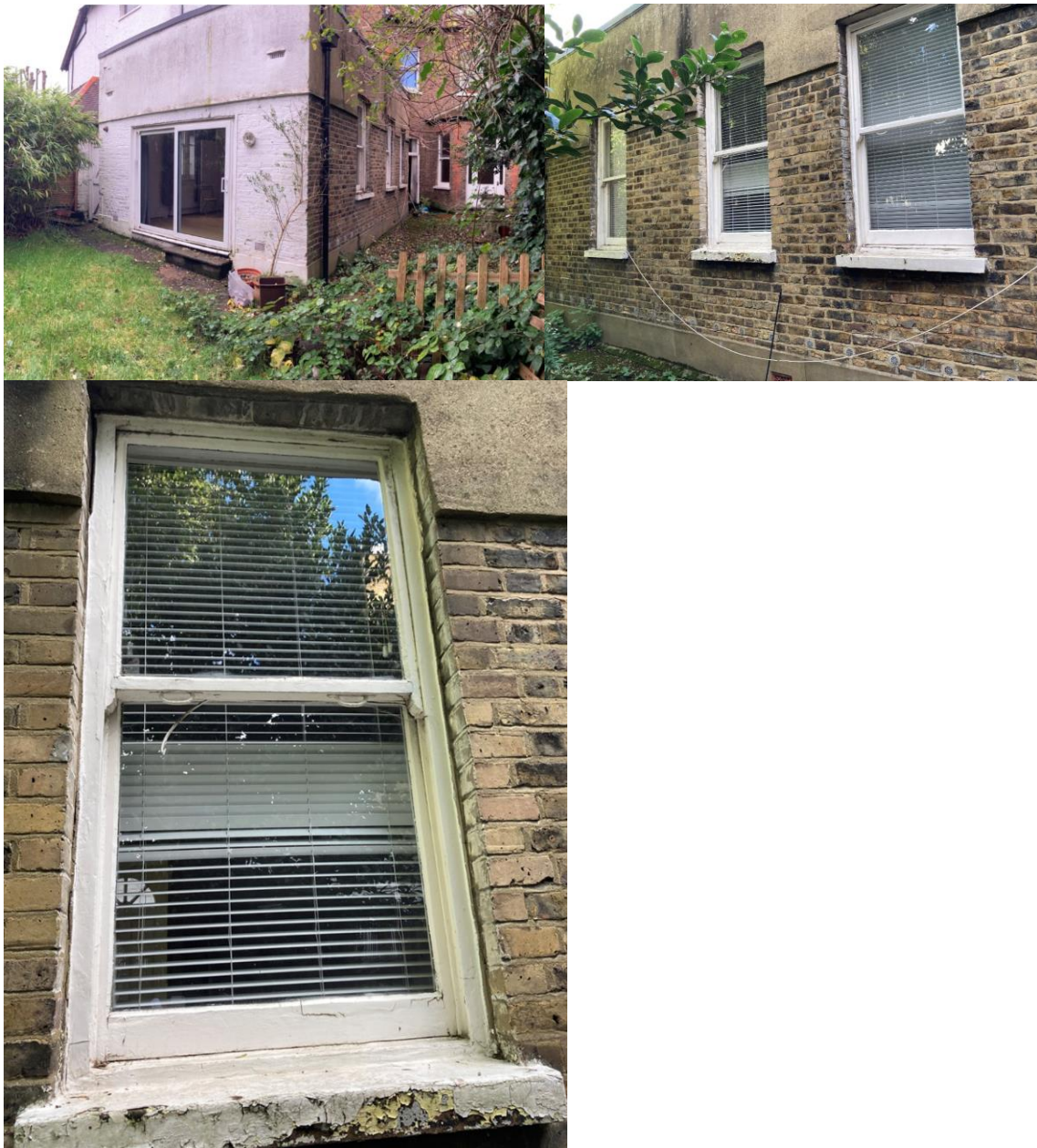
Above: Existing rear and side elevation windows and doors. The existing timber windows are in need of renewal due to their poor condition, with rotting and crumbling timber
