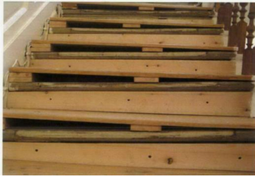
Figures 9: Photograph of the works carried out to the staircase following the 2004 consent.
