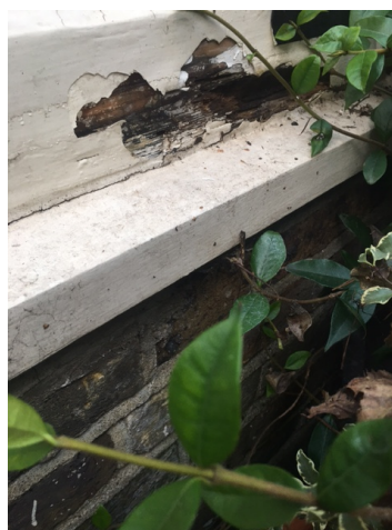
wood rot on bottom sill
