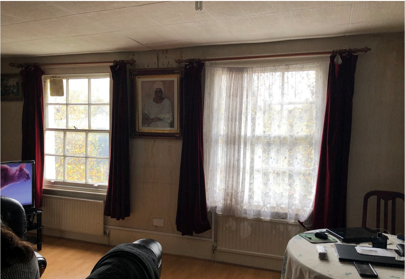
Figure 4: Internal view of sitting room windows at second floor level (Flat C)
