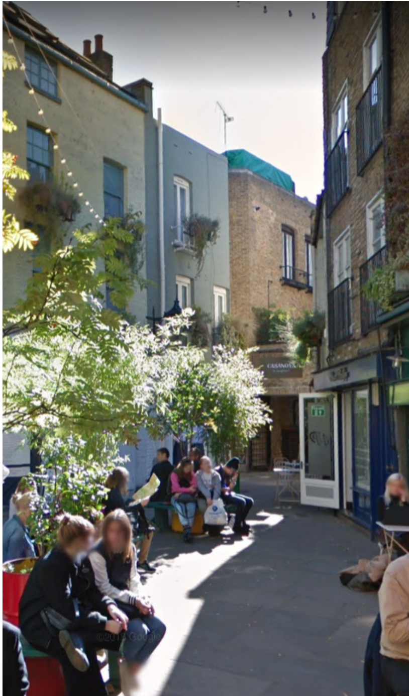
Photo 3 (above): Roofline of 3 Shorts Gardens as viewed from Neal's Yard. The existing plant enclosure is shown covered by a green tarpaulin
