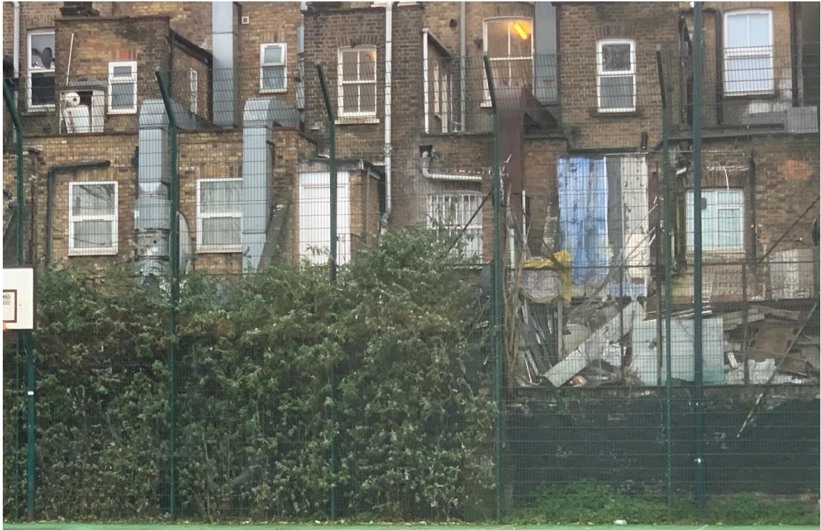
Picture 10: Rear of 284 Kilburn high road showing unwanted plant growth & damaged boundary wall (similar condition to previous rear wall of property)
