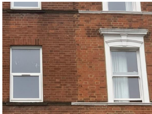
Picture 2: Contrast in window detail with neighbouring property
