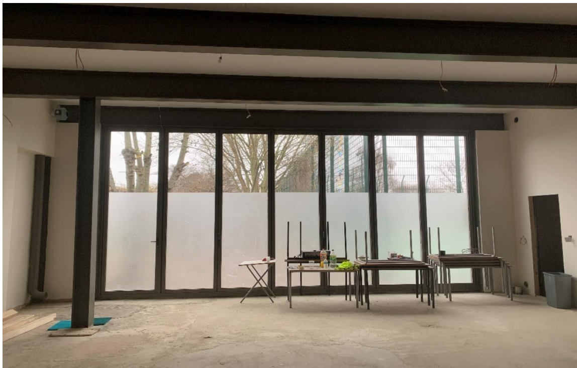
Picture 11: Internal view of bi-folding glazed doors with from main hall (2.2m high obscured glazing)
