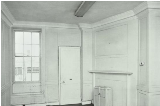
A view of a second-floor rear room at 8 Great James Street in 1976, [71891]
