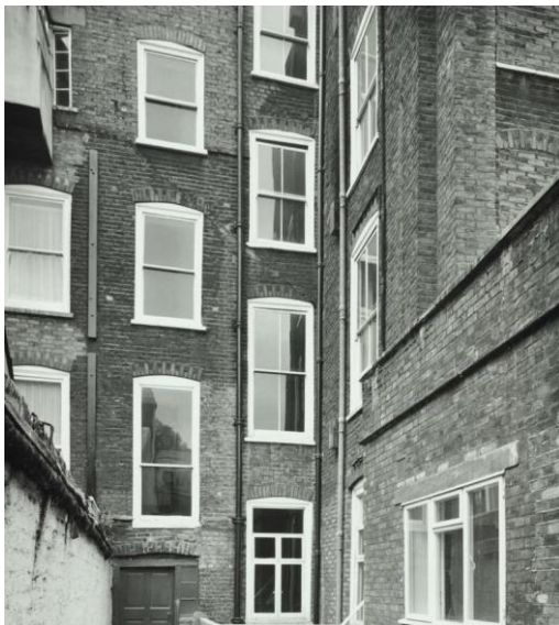
Figure 13: A view of the rear elevation of No. 7 Great James Street in 1976. Lower outbuildings also seen. [© LMA Collage Collection, image no. 71898]
