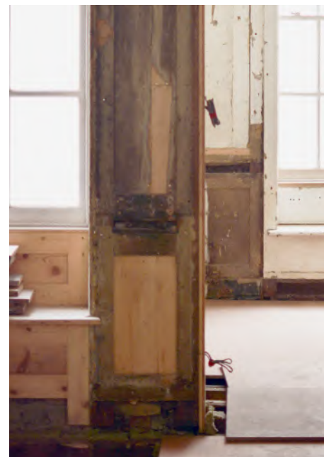
Restoration of wall panelling at 34 Great James Street with piecing in where required
