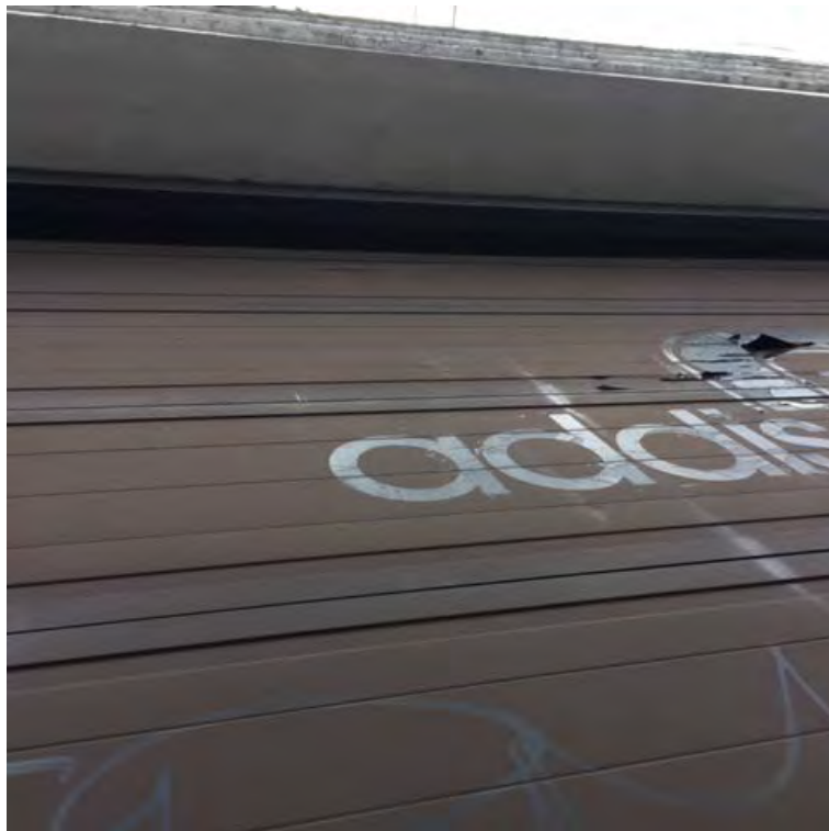
Photograph 4 – Gaps under roller door
