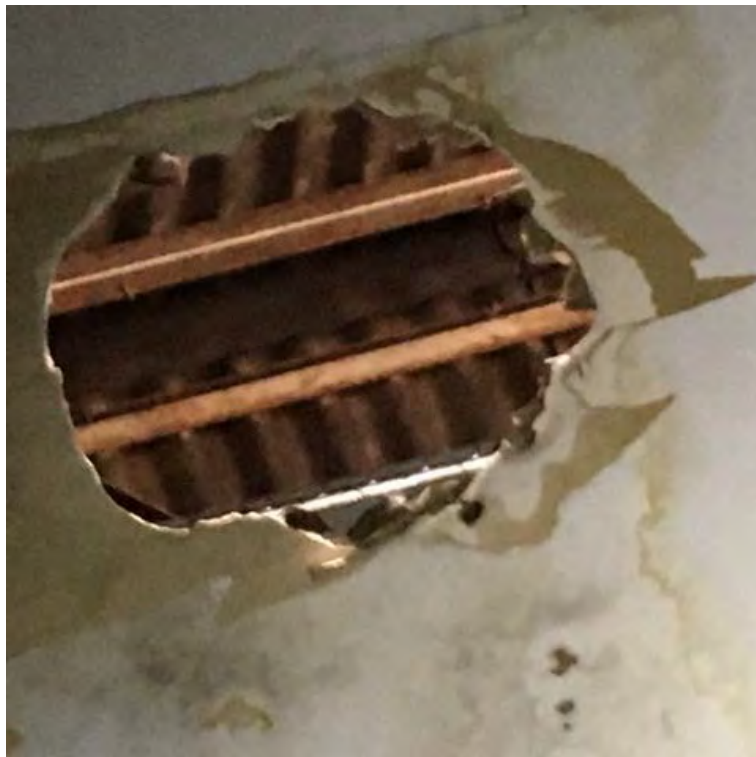
Photograph 6 – Holes in ceiling showing overlapping metal sheeting
