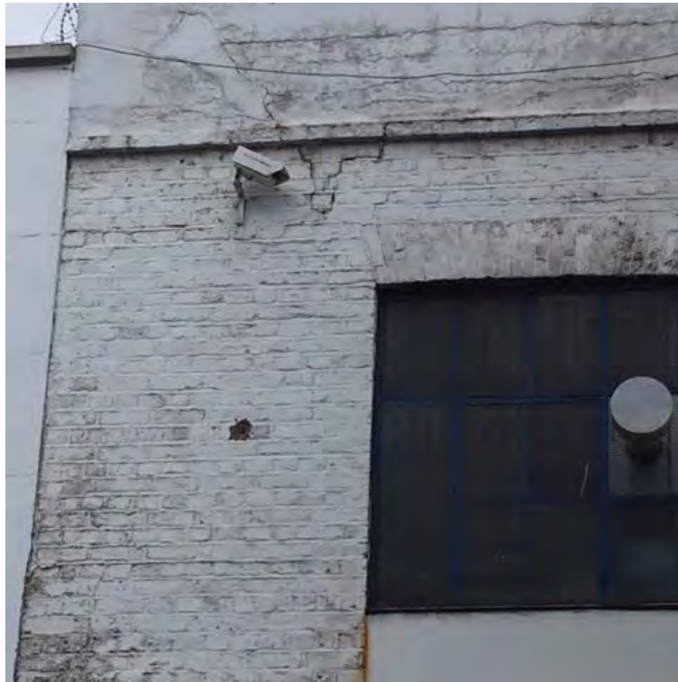
Photograph 3 – Superficial cracks in brickwork
