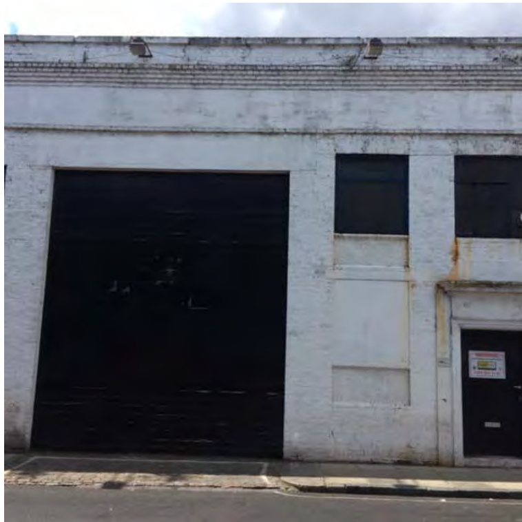
Photograph 2 – Lighting on north-eastern aspect of B1
