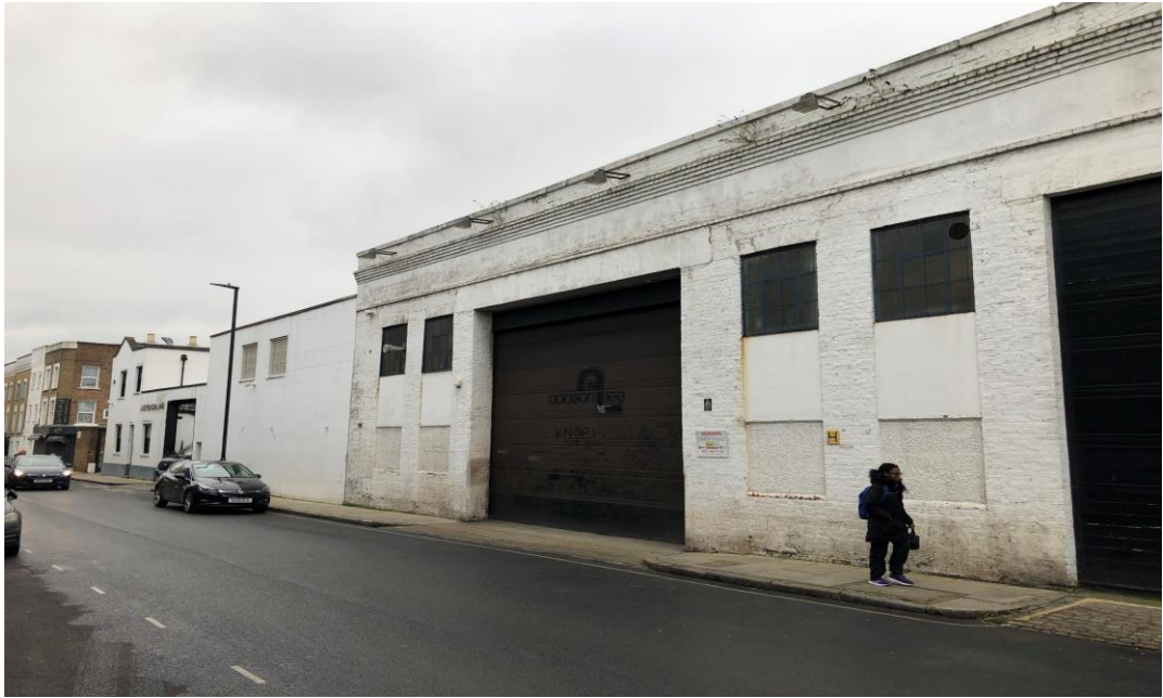
General view of existing elevation showcasing begrimed painted masonry and spalling areas of render.
