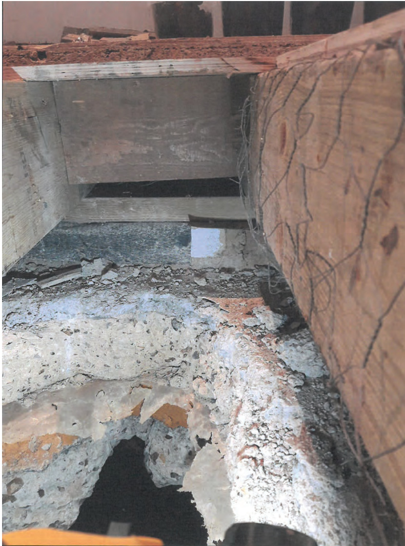
Photograph of "Trial Pit 2". The "upper slab" can be seen in timber construction. The "lower slab" can be seen below with plastic DPM below. A large void is also visible at the bottom of the photograph.
