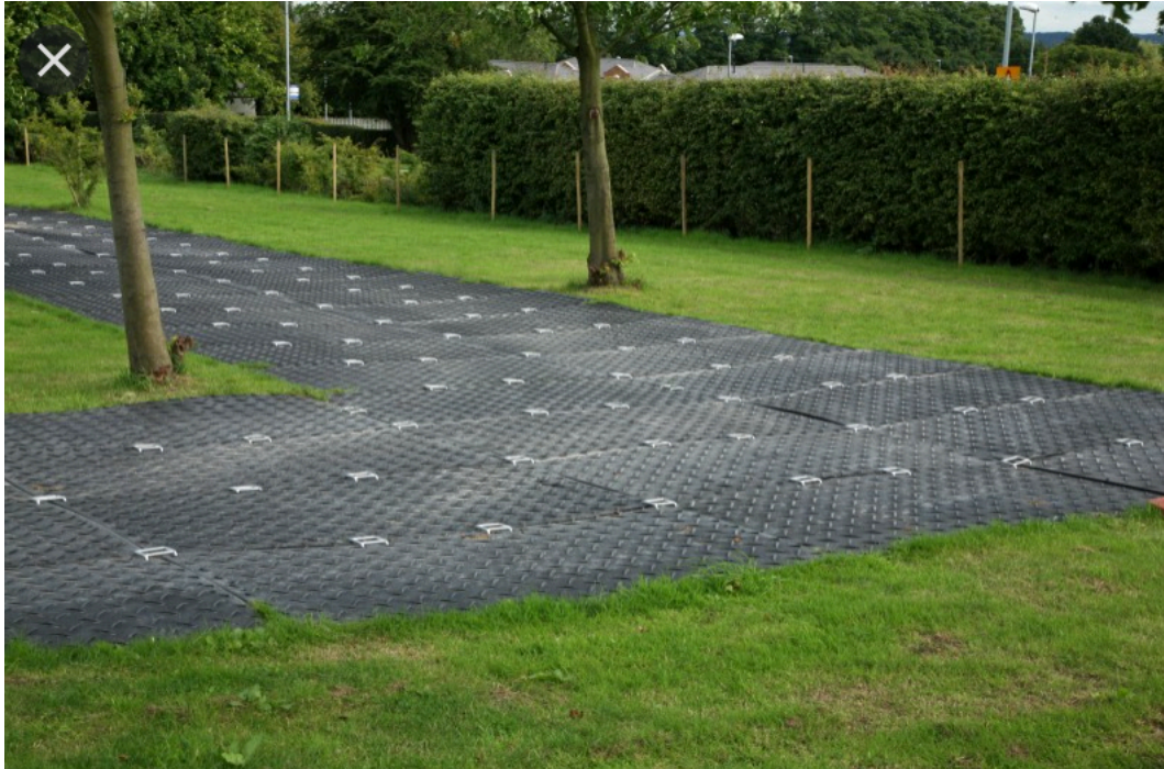
Photograph 1: Example of ground protection using Ground Guards Interlocked over 100mm mulch base layer
